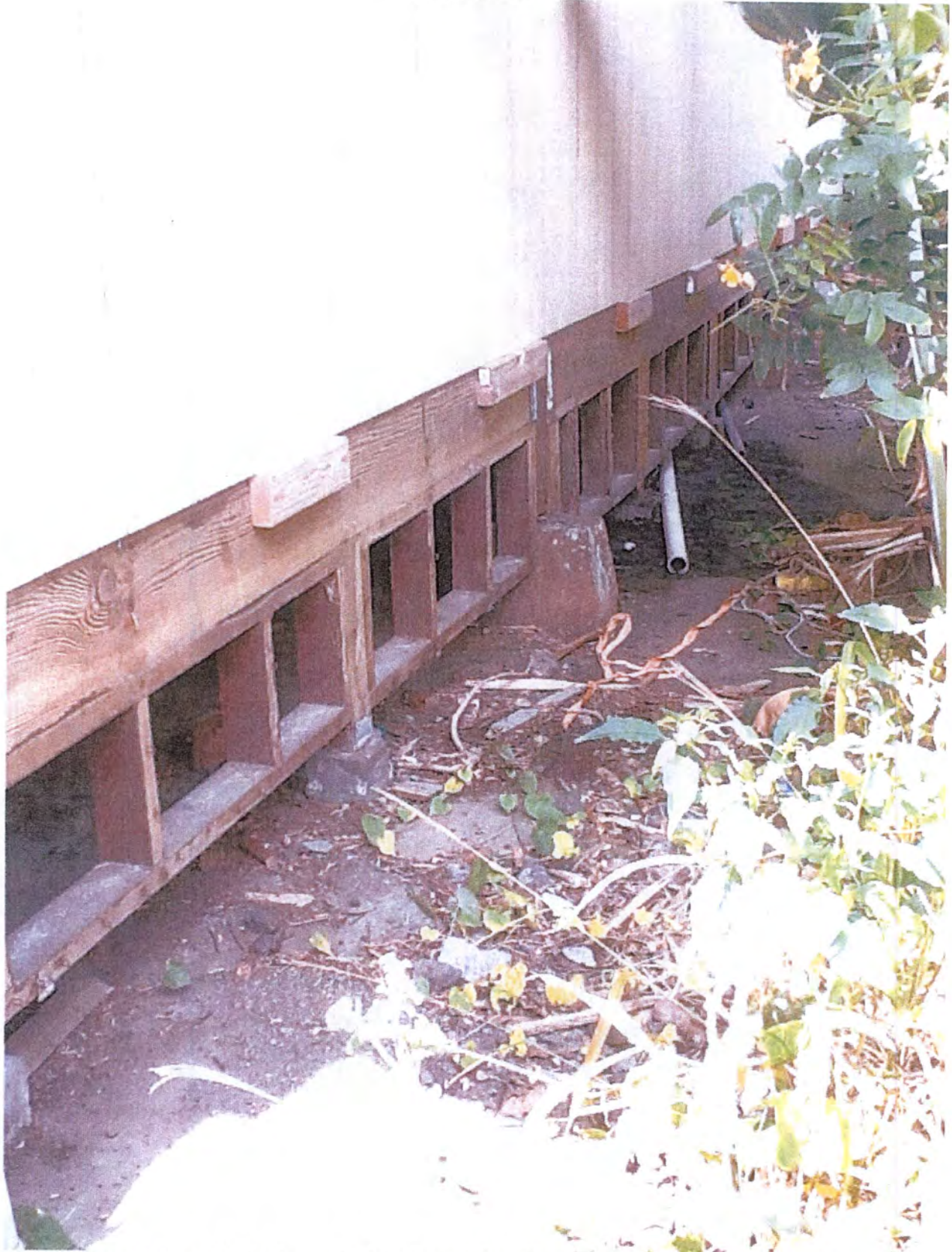
Depicts the cripple wall that is parallel to the neighboring property from which the photographs were taken. Note the pipes from which liquid appears to be leaking.
